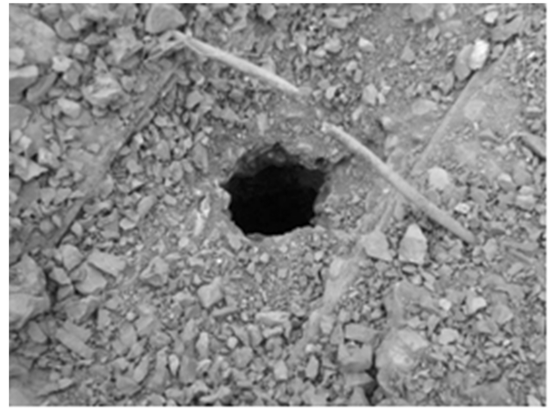
图 7 实验后靶标 Fig. 7 Reinforced concrete after experiment
