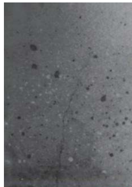
(e) Shear crack 1
