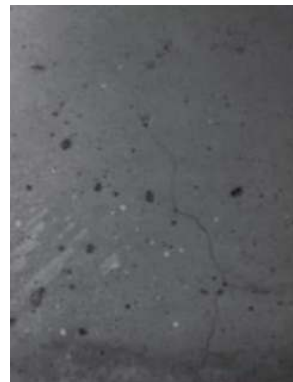
(f) Shear crack 2
